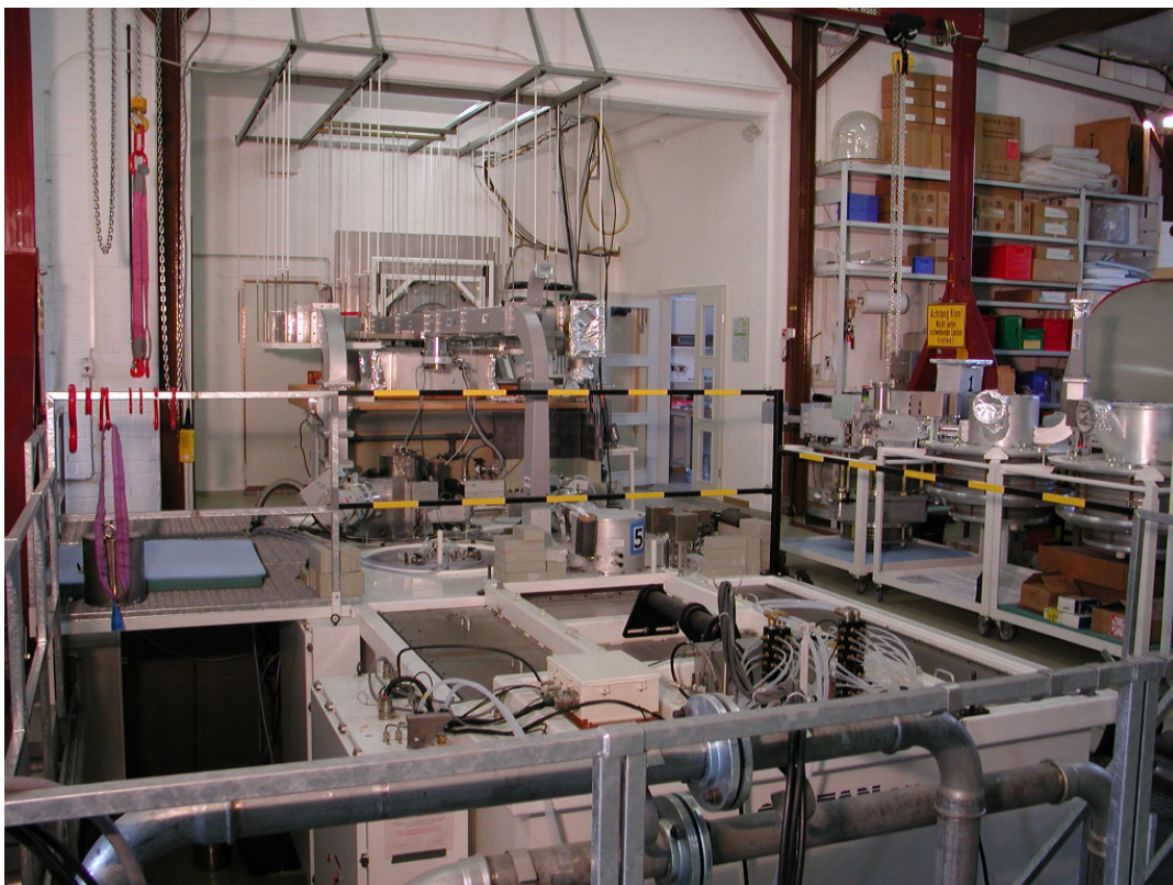
Figure 1: HPM system with new tube 5 and shunt installed, and tube 3 (idle)
