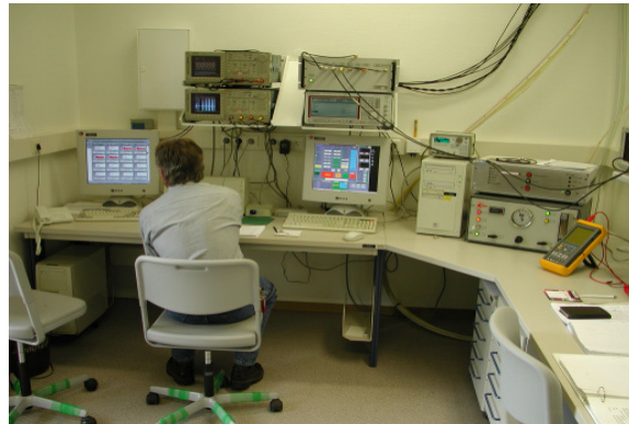
Figure 3: Control room with control units and data acquisition system
